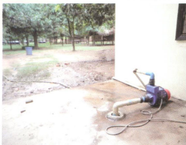
Water from covered well
