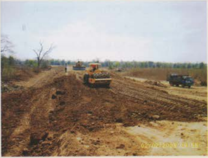
H.E Lim Kean Hor, monitored spillway structure of Kampong Chrey Irrigation System
